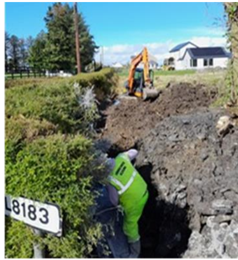
ALLEVIATION OF SURFACE WATER ISSUE AT GALBOLEY, BULLAUN, LOUGHREA AFFECTING THE LOCAL ROAD BUT INVOLVING A CROSSING OF THE REGIONAL ROAD
