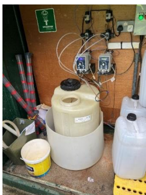
NEW CHEMICAL DOSING SYSTEM AT KYLEMORE ABBEY TO REDUCE PHOSPHORUS DISCHARGING TO THE SENSITIVE DAWROS CATCHMENT
